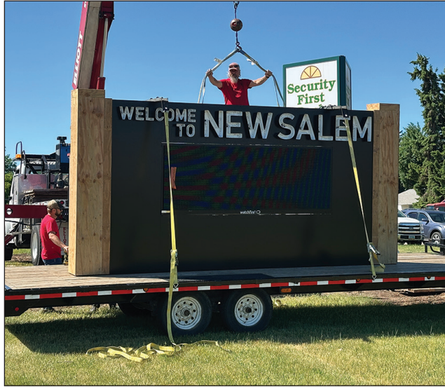
photo | Richard Mendoza INSTALLATION of the new welcome sign and digital messaging center, which will be located on the grass in front of Security First Bank, has taken place. The project is a collaboration between Security First and the New Salem Betterment Committee.
