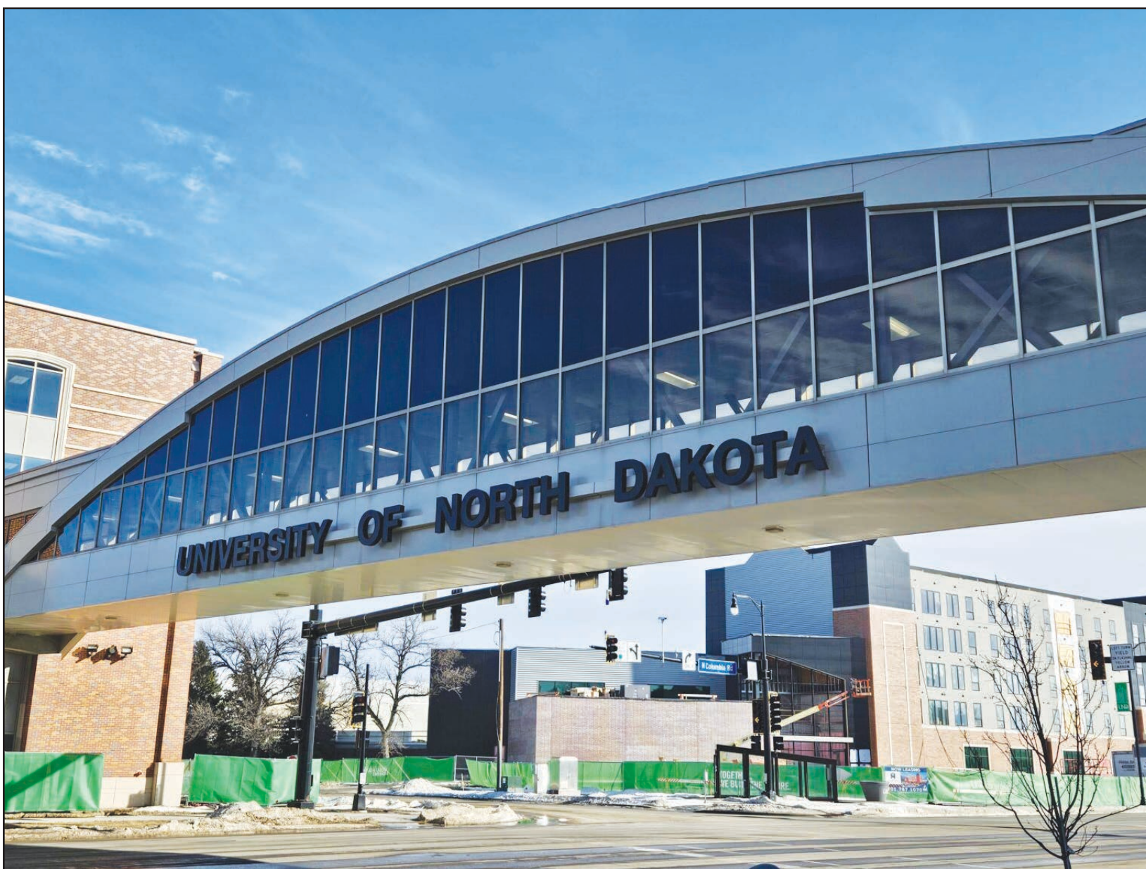
A construction project was in progress on March 1, 2024 on the University of North Dakota campus in Grand Forks. (Photo by Jeff Beach / North Dakota Monitor)
