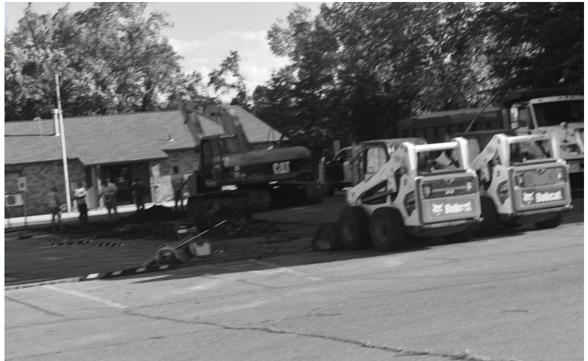
PHOTO CREDIT OF DANIEL ARENS Keller Paving out of Minot does asphalt patching and repair work around town, including at the Hazen Senior Center on June 15. Several problem spots for asphalt were identified by the Hazen City Commission to be included in a summer project this year.
